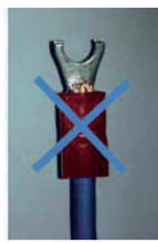
Terminal has been cut.
